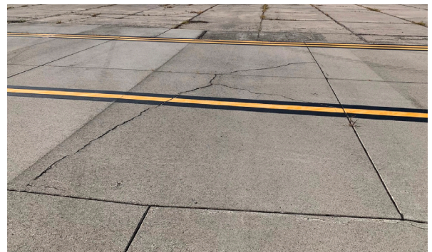
Crack in Aircraft Parking Apron Asphalt Surface
