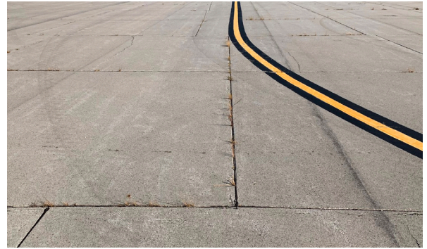
Aircraft Parking Apron with Vegetative Growth
