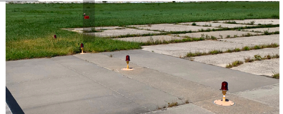
Runway 17 Threshold Lights
