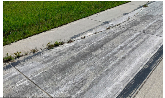
Cracked Panels at Runway 17 End
